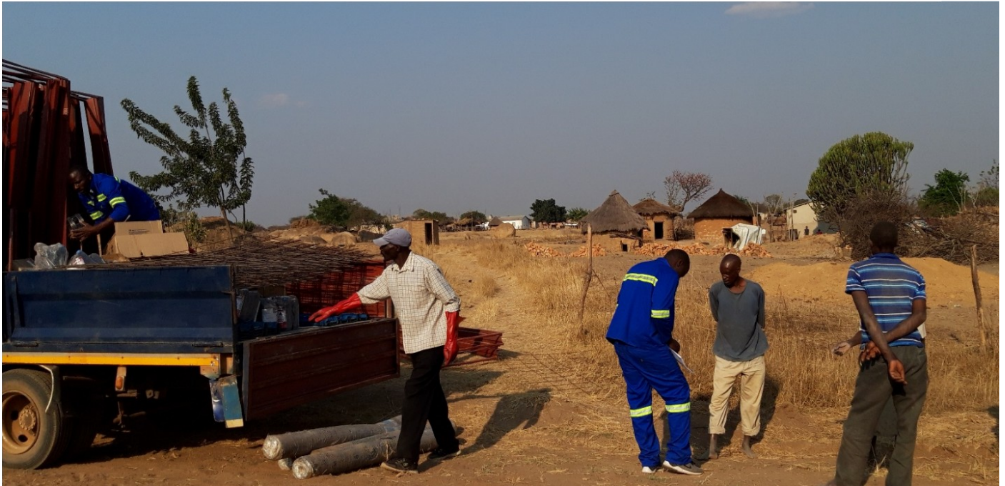
Distribution of building materials to beneficiaries of the shelter component who are ready to start construction with all locally found materials mobilised. On picture distribution was taking place in ward 17, Rufu village.
