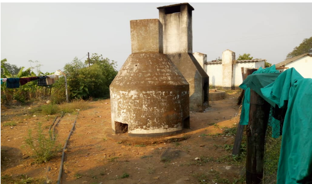
Assessments of waste zone at Mutsvangwa clinic Chimanimani in ward 23 The solid waste management site was selected for rehabilitation.
