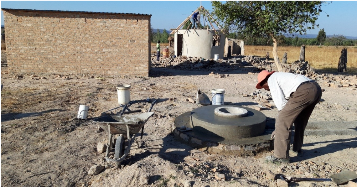
Deep well at Mr and Mrs Paradza Unyai's homestead. The new deep well was constructed by a local builder.
