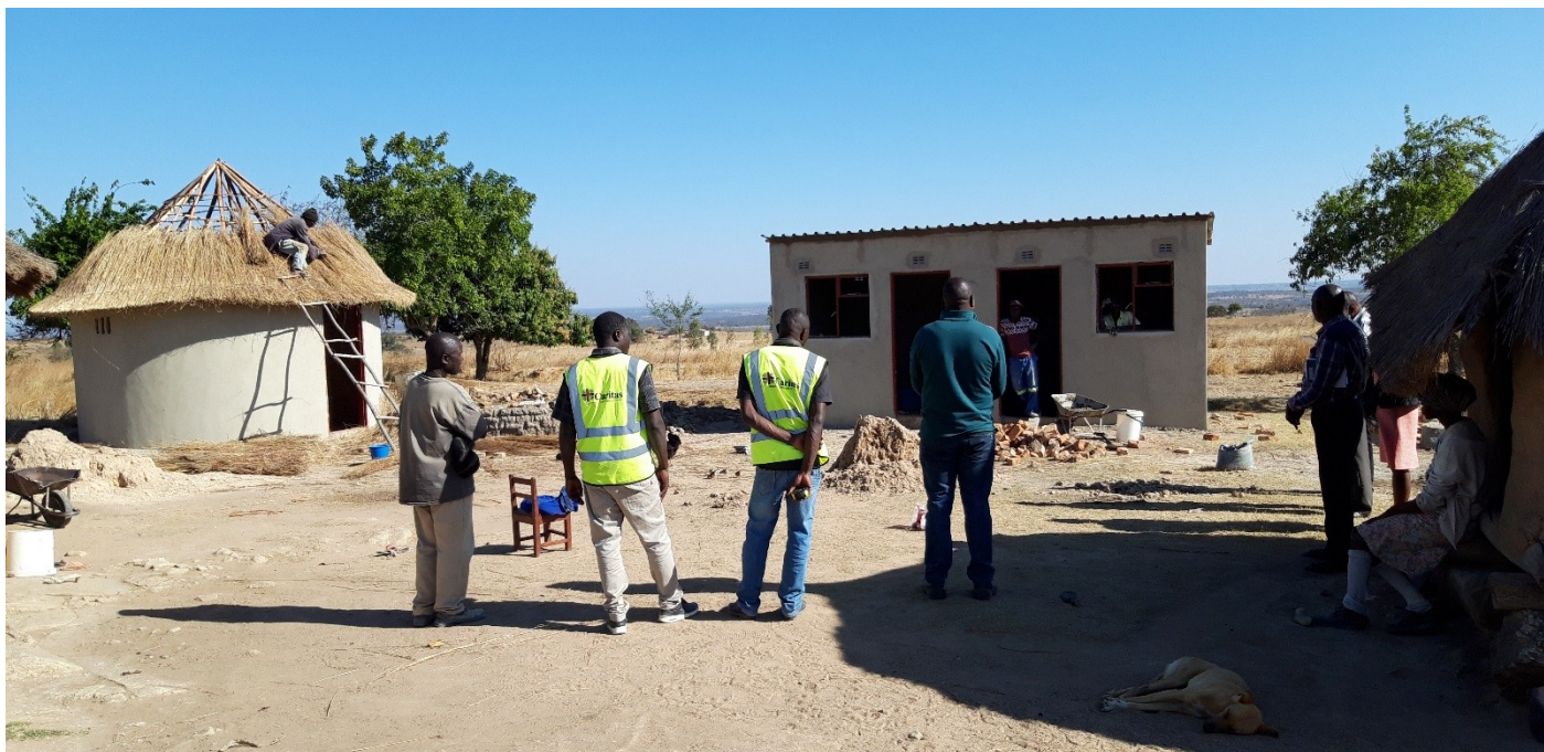
Ms Shindi's homestead nearing completion during the monitoring visit by CAFOD (Mr Mashiri) AND Caritas National office (Mr Dzveta). Thatching in progress using the grass mobilised by Ms Shindi (picture above). The construction was conducted by local builders and thatcher.
