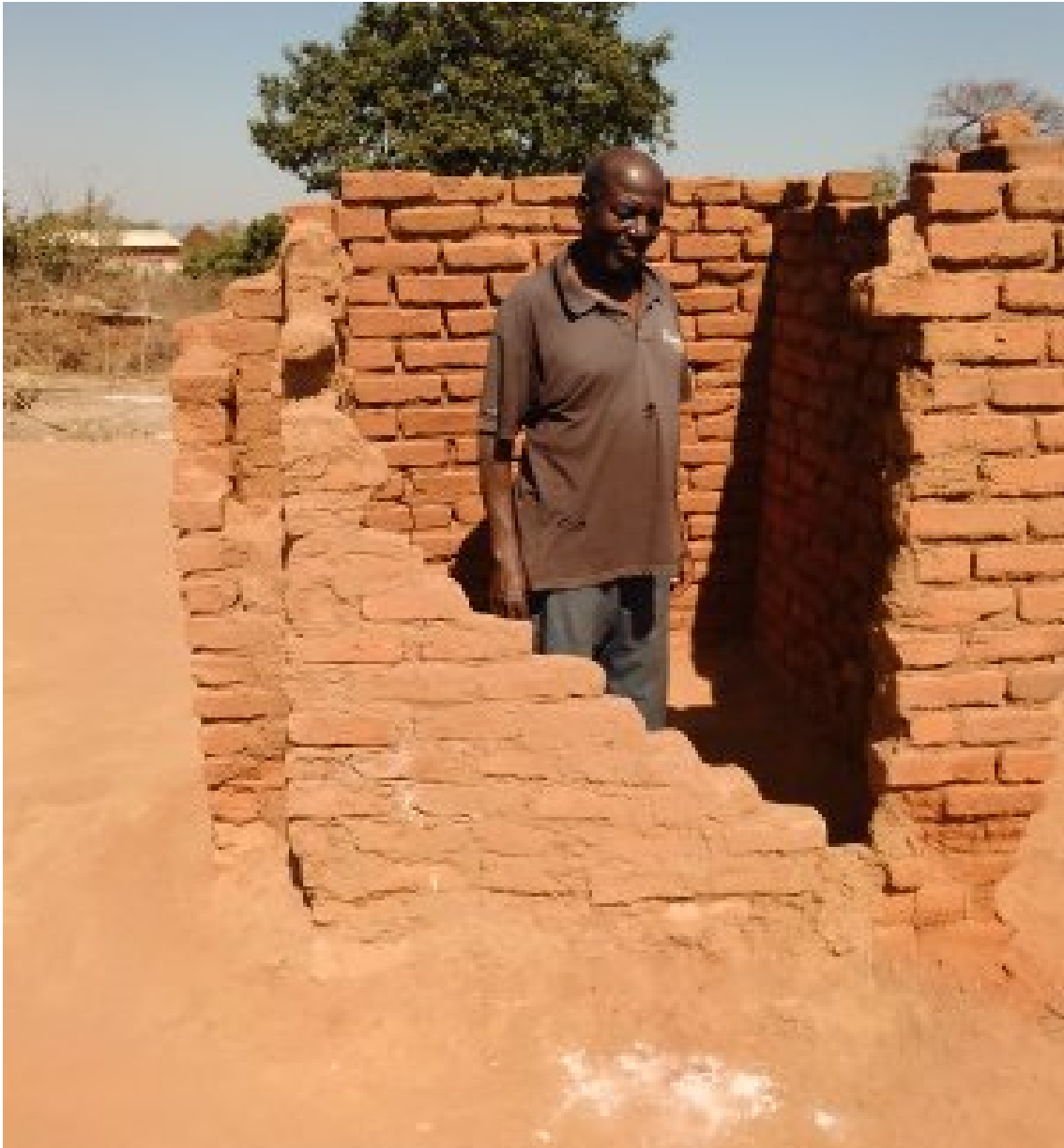
Toilet beneficiary observed inside the toilet destroyed by cyclone Idai in Ward 22, Gangarabwe of Bikita district
